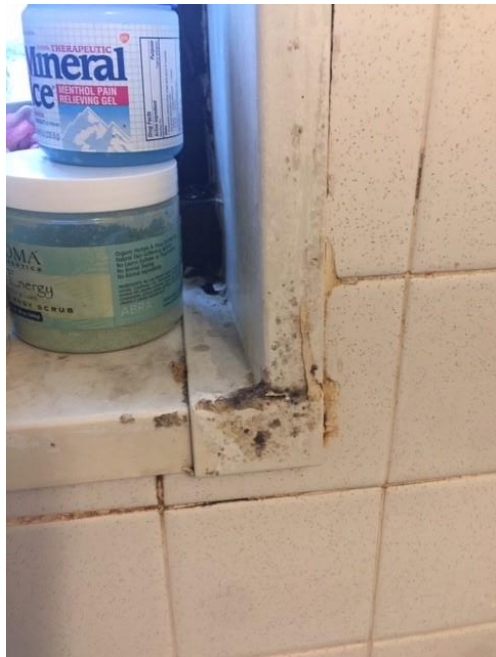
Close Up: Bathroom Window Frame
