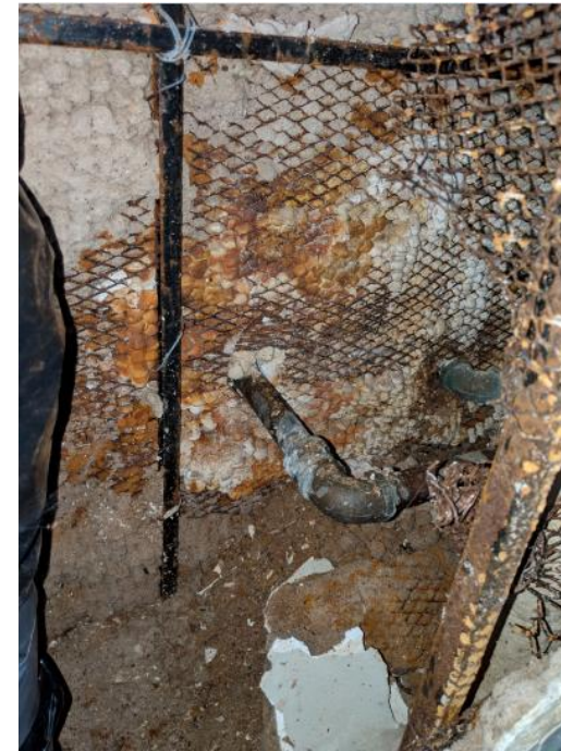
Missing insulation on cold water supply t
