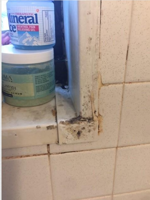
Close Up: Bathroom Window Frame
