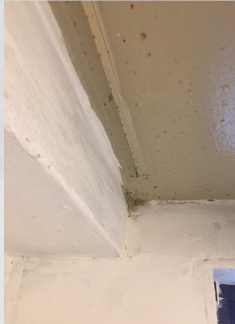
Close Up: Bathroom Ceiling
