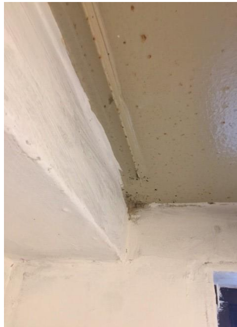
Close Up: Bathroom Ceiling
