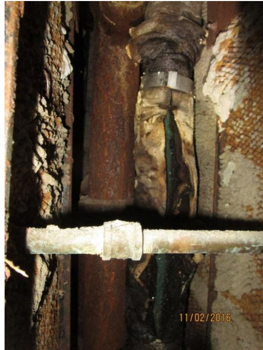
Damaged insulation on cold water riser
